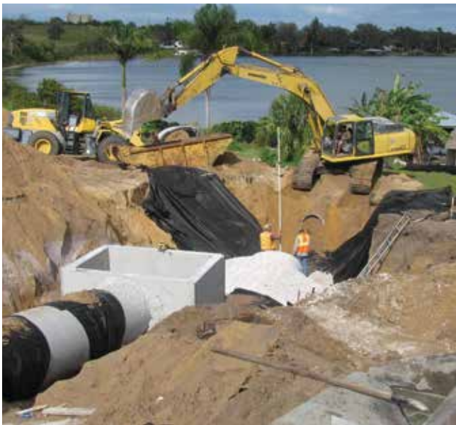
An excavation point crew installs downhill stormwater system components for the Lake Clay Stormwater Retrofit system on the West Coast of Central Florida. Credit: Highlands County Natural Resources Department
